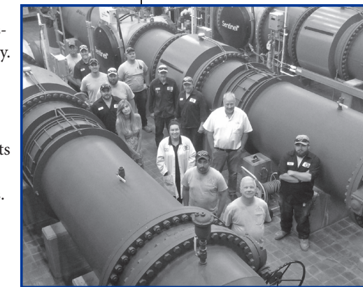
Delivery Quality – Day side staff in UV room at Three Rivers Water Filtration Plant
